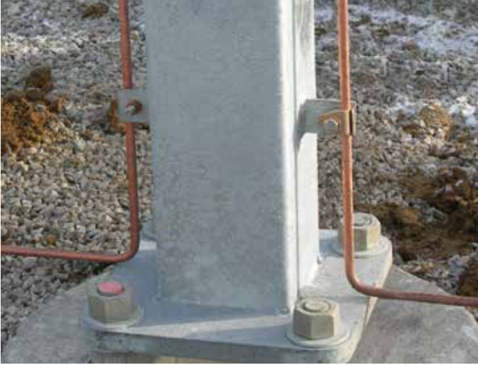
Substation earthing riser
