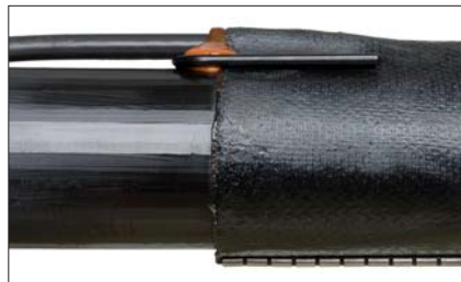
Shield break connection
