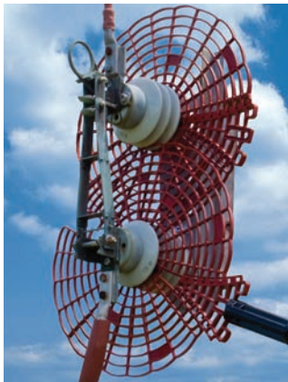
BISG-24 energized install
