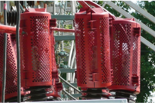
BCAC-IC Installed on Bushings
