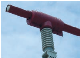
2 Pieces: MVLC-38 on busbar with BCIC
