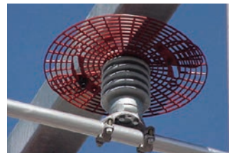
BISG-60/115-02 installed on bus support insulator
